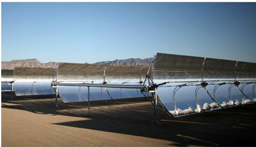
Parabolic-trough collectors in the Nevada Solar One power plant Source: Taylan and Berberoglu, Fuel Production Using Concentrated Solar Energy , accessed on April 22 nd , 2021
