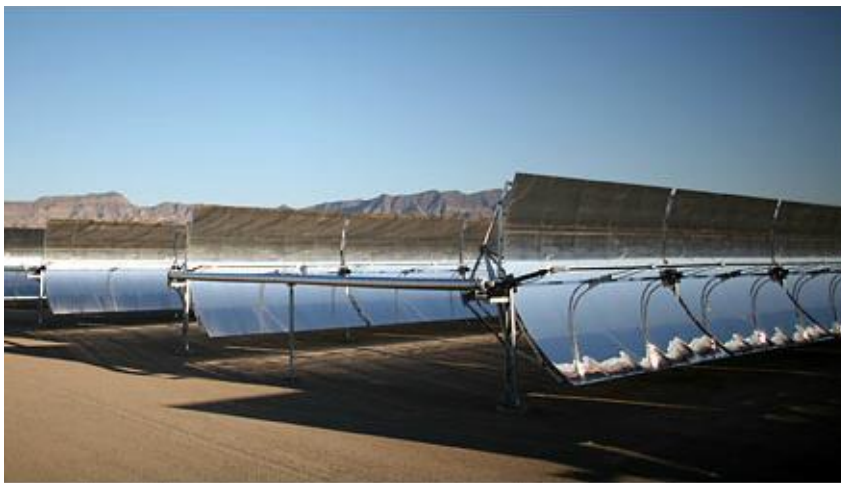
Parabolic-trough collectors in the Nevada Solar One power plant Source: Taylan and Berberoğlu, Fuel Production Using Concentrated Solar Energy , accessed on April 22 nd , 2021
